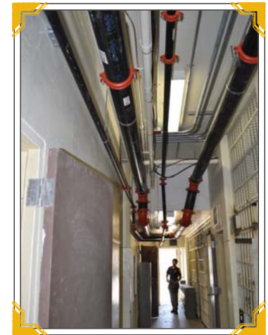
Construction contractors installed pipes and sprinkler heads in 100% of the Newport News City Jail.
