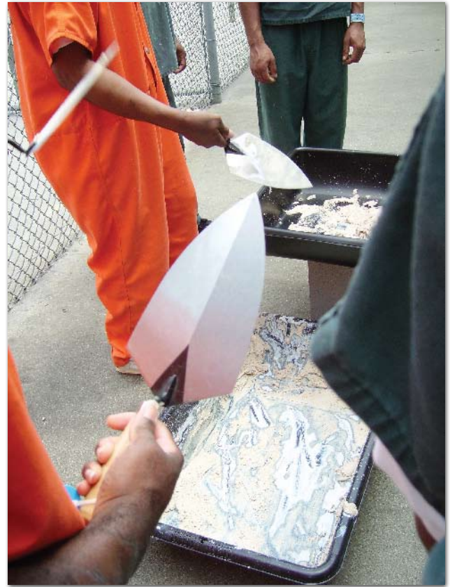
Before setting their trowel into mortar, inmates first get a feel for the finesse of handling the tool.
